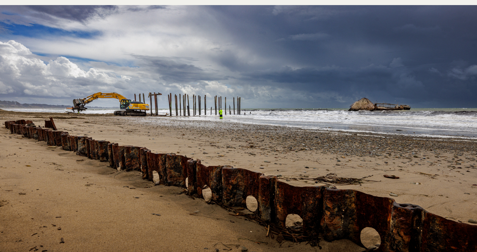
The pier at Seacliff State Beach was demolished after suffering damage during the January 2023 storms / Kevin Painchaud
