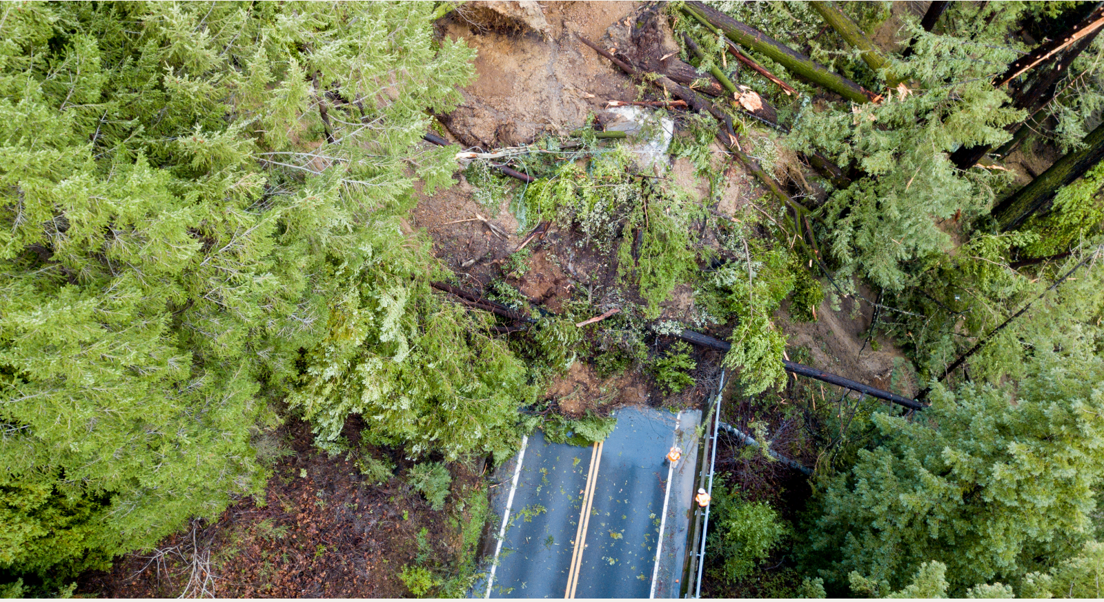
Aerial footage of a massive landslide on Highway 9 in Ben Lomond/ Kevin Painchaud
