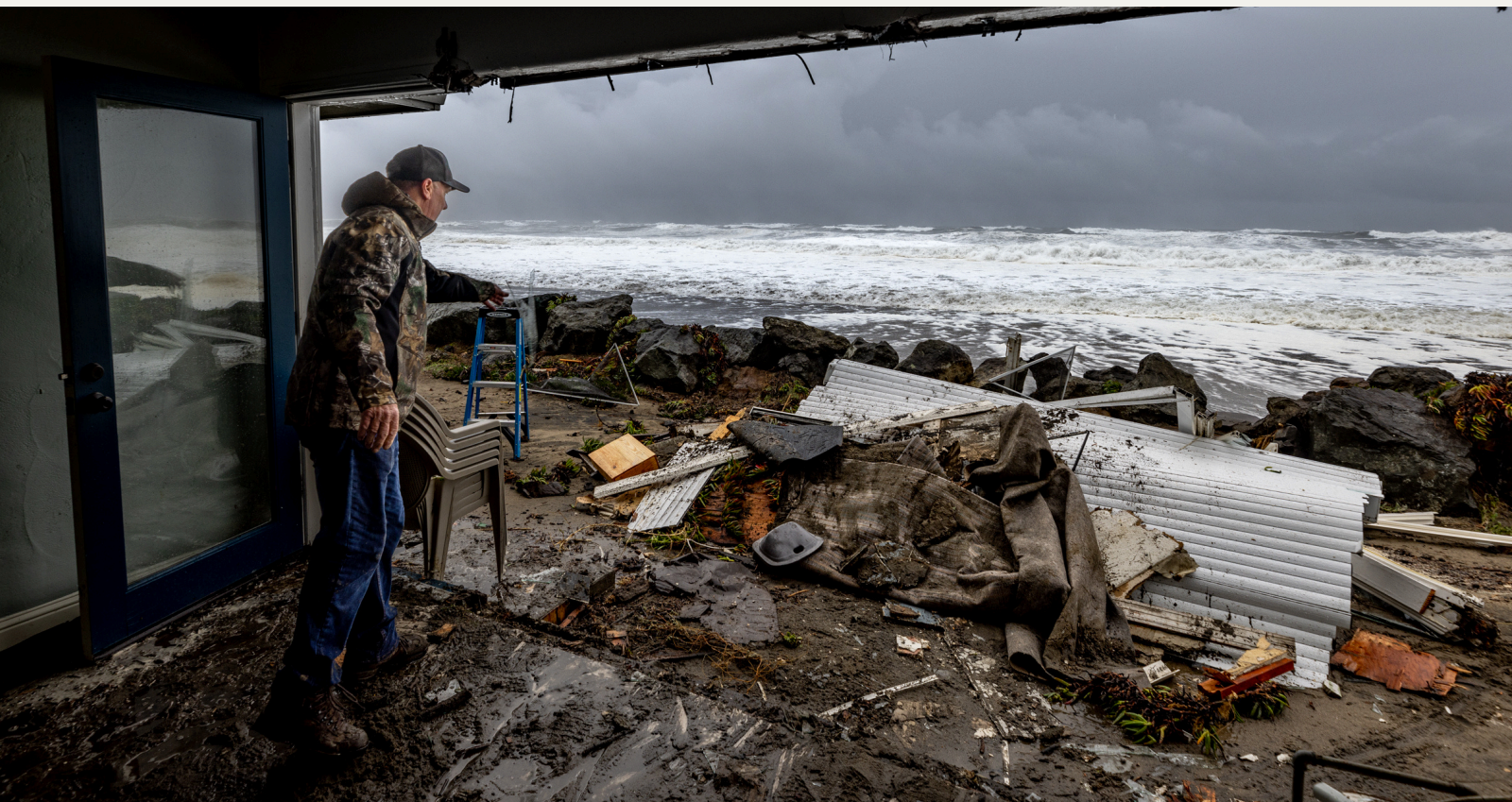
Ocean swells knocked out the front wall of Eric Stark’s oceanfront home in Rio Del Mar on Jan. 5 / Kevin Painchaud
