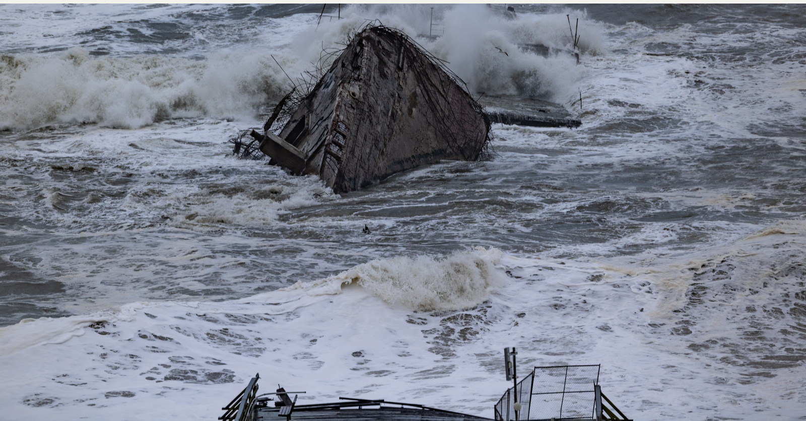
The damaged pier at Seacliff State Beach that led to the beloved Cement Ship on Jan. 5/ Kevin Painchaud
