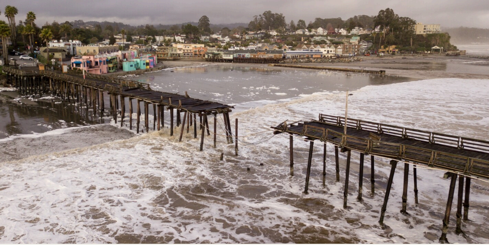
Aerial shot of the damage to Capitola Village and pier on Jan. 5 / Kevin Painchaud
